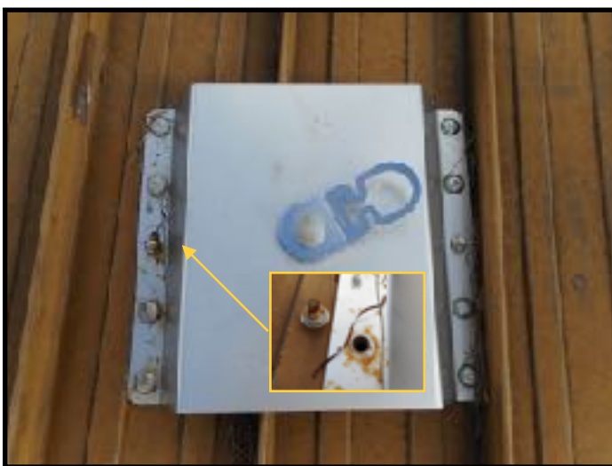
Product Failing Inspection
